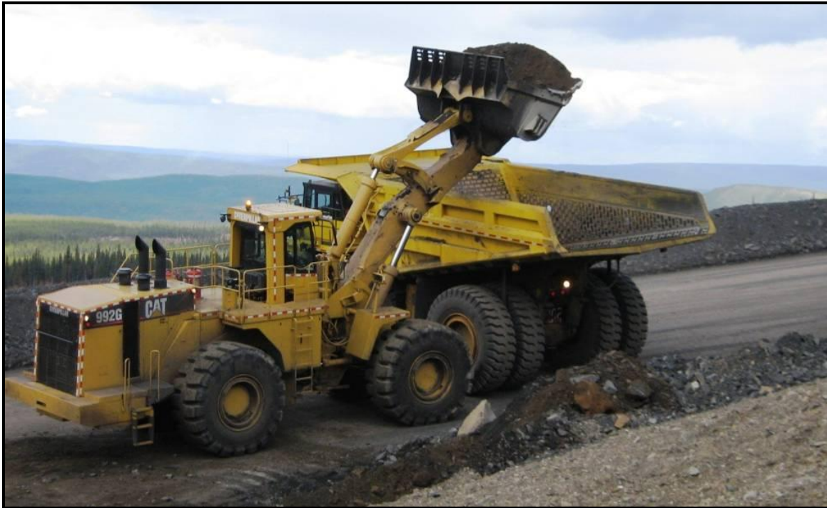
Truck operator backs truck in square to the loader, directly under the bucket.
