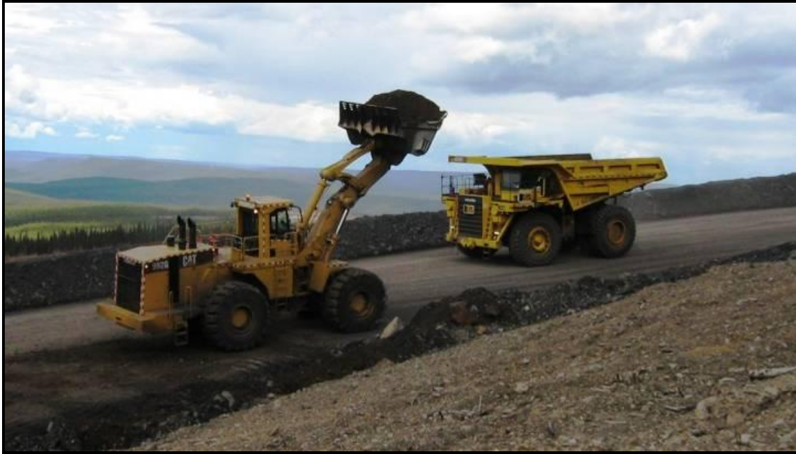
Truck approaches front-end loader from the left side. Loader operator uses his bucket to guide the truck.
